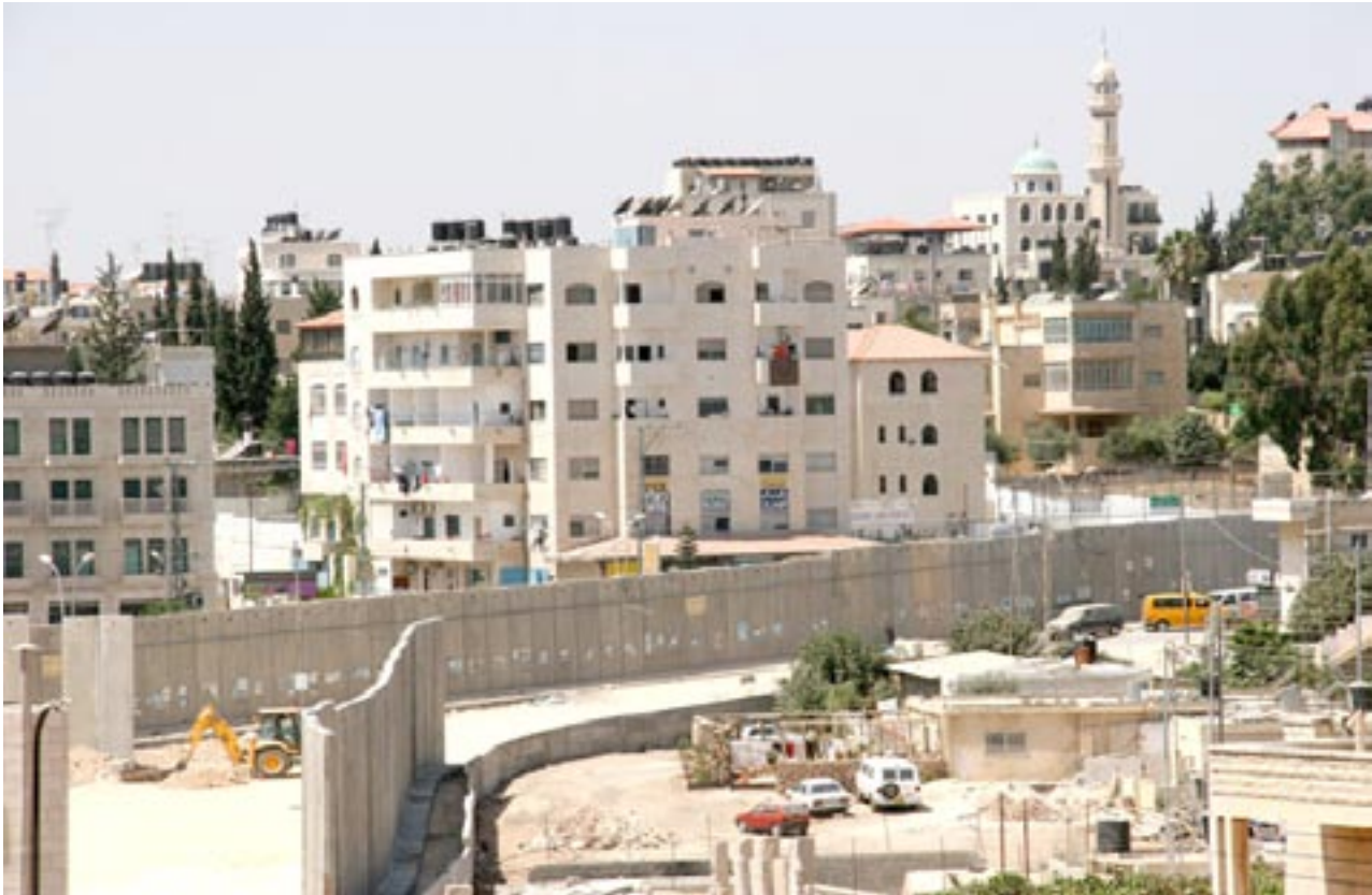
Al-Ram, the construction of the Wall, which is located on the main street and passes through the neighbourhood, August 2006. © Anne Paq.
