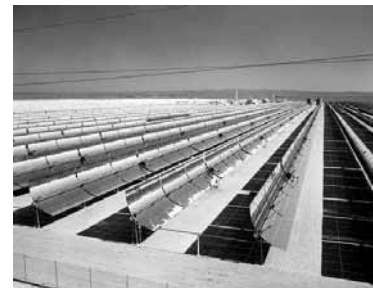
Fig. 3-8: One of nine solar electric energy generating systems at Kramer Junction, California.
