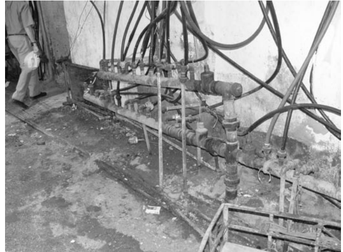
Figure 3.2: Water pipe connections to main- Burj El Barajneh
