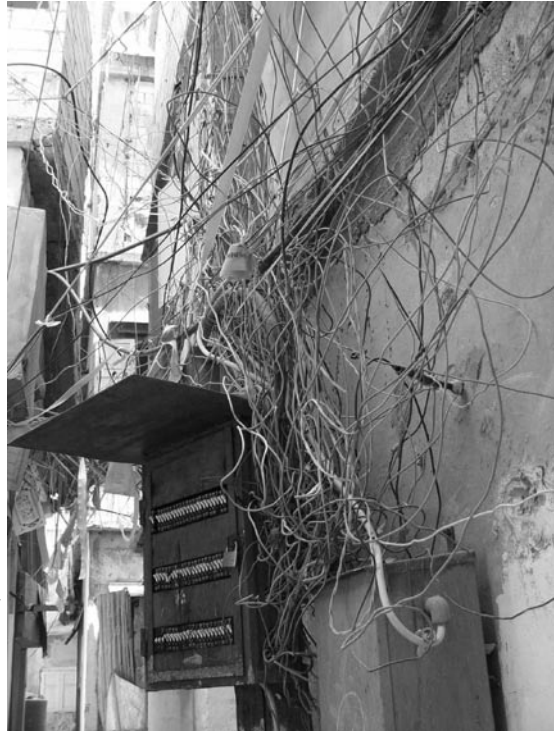
Figure 3.3: Electrical wires tapping into a power main- Burj El Barajneh
