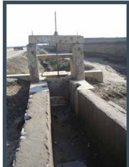
Illustration 23: Tertiary control gate, Parwan scheme (Bob Rout photograph)
