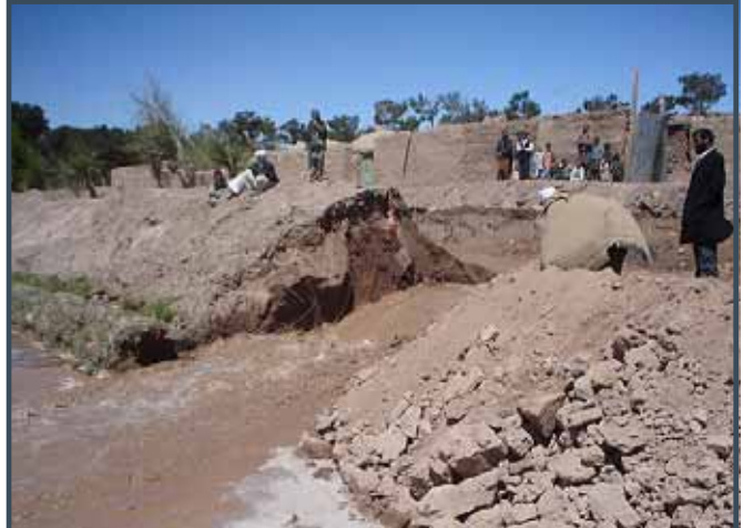
Illustration 7: Breach in main canal (April 2005)
