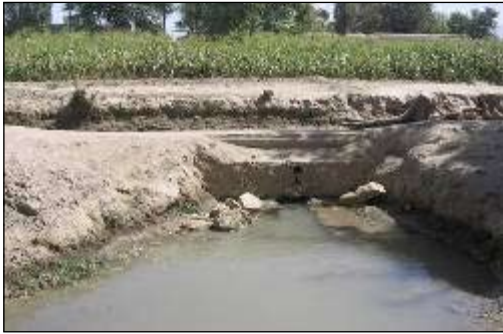
Photograph 1: Zahir Janan offtake (concreted during Sugar Factory period)
