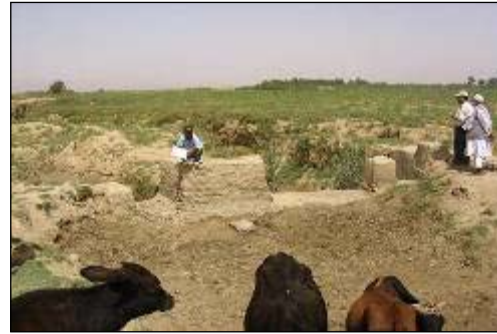
Photograph 2: Cimeti offtake (concreted during Sugar Factory offtake). On the right side, the main canal is dropping (~2 meters).
