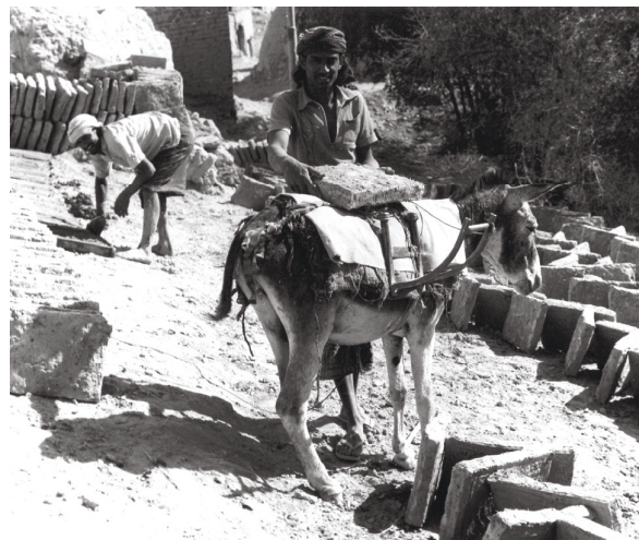
Figure 70. Transporting mud bricks. Donkey pack saddle with modern “wings” of metal pipes (cf. figure 36).
