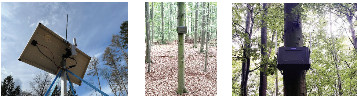
Figure 14: Solar-powered LoRaWAN gateway with internet access and the LoRaWAN GW2ED Range Extender located in a forest in Wolfenbüttel, Germany.
