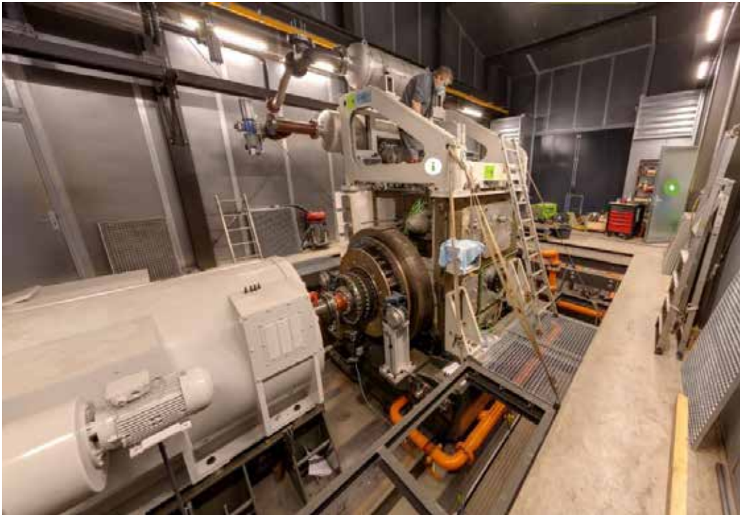
Figure 10 - Single Cylinder Engine Testbench
