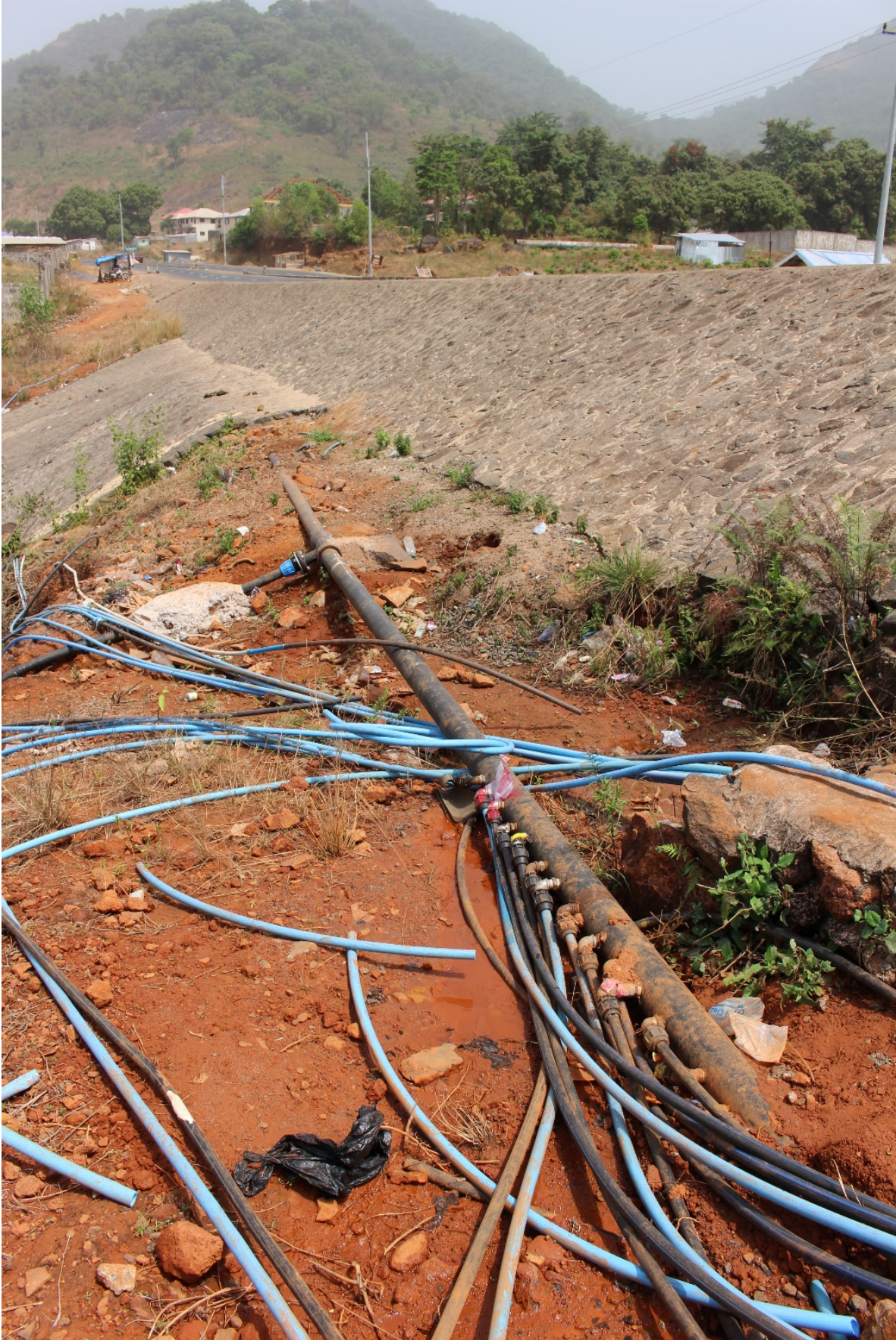
Figure 4.2.: Spaghetti connections on a sub-main (photo taken by Lorenz Gosch)
