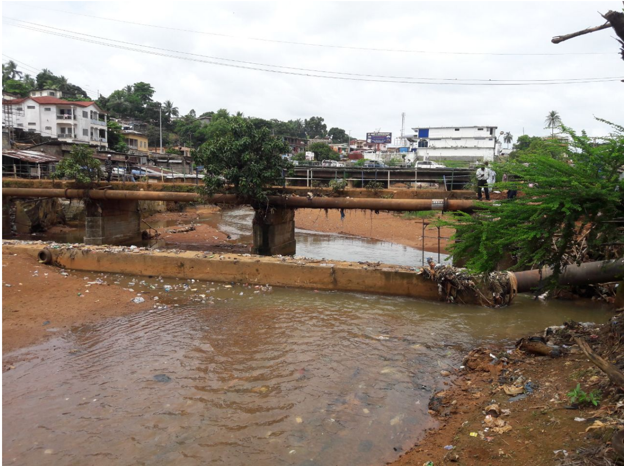
Figure 3.2.: Juba Bridge with the two main transmission lines (photo taken by Lorenz Gosch)
