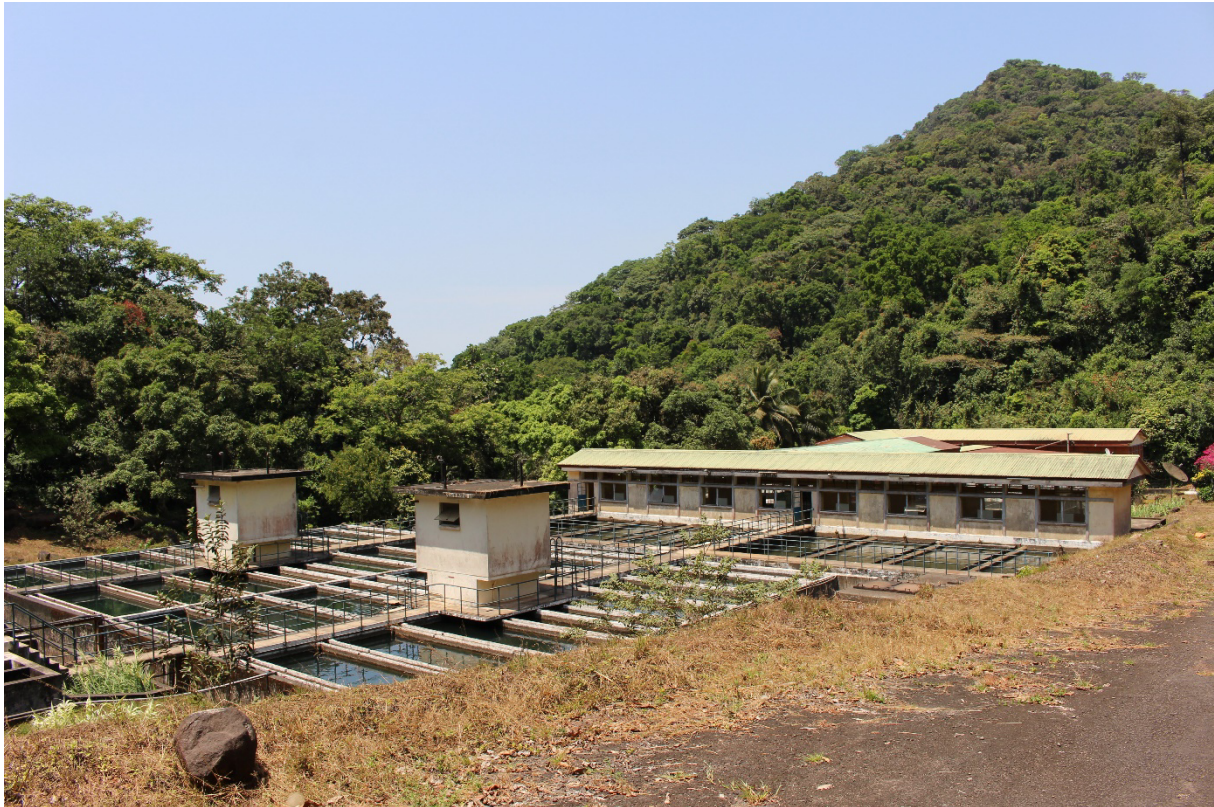
Figure 3.1.: Guma's water treatment works (photo taken by Lorenz Gosch)
