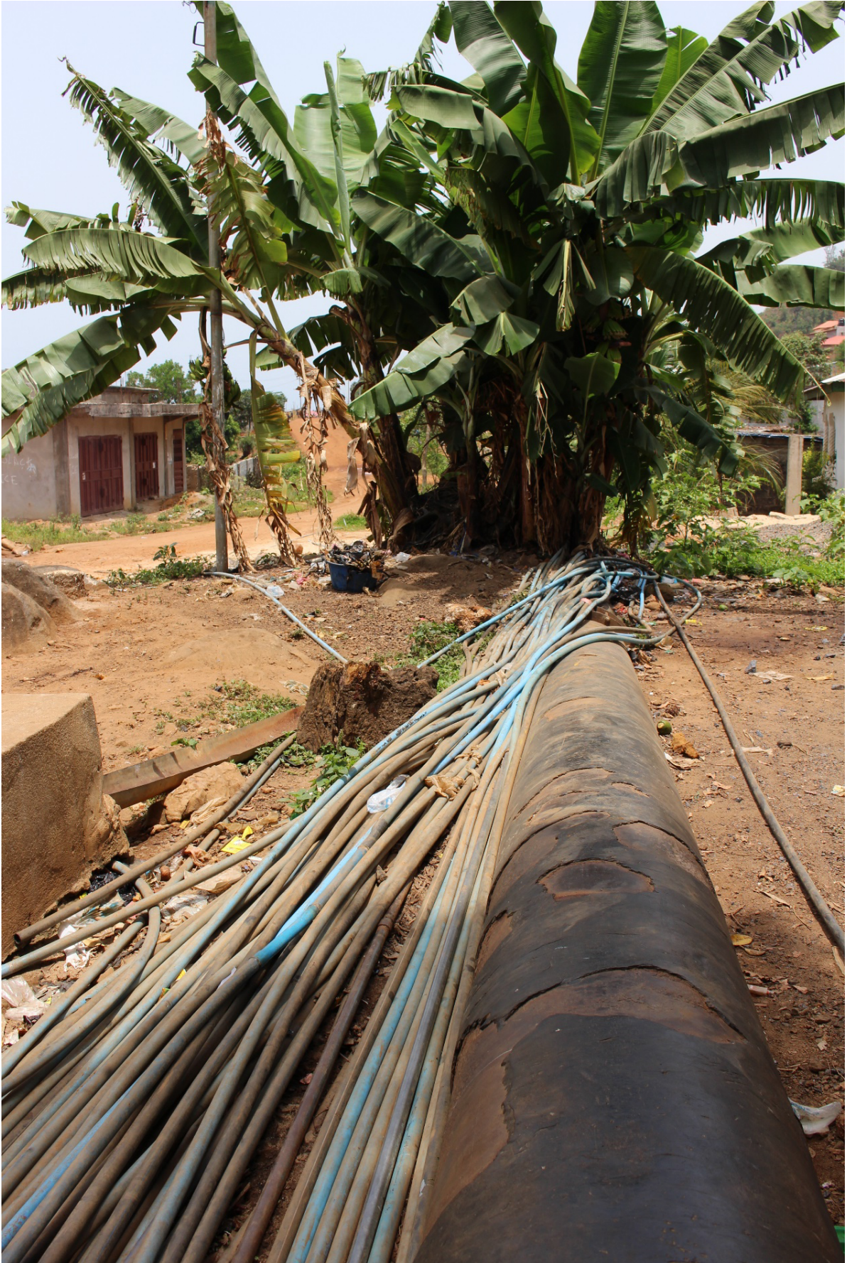
Figure 4.1.: The 18-21inch main being accompanied by "spaghetti pipes" (photo taken by Lorenz Gosch)
