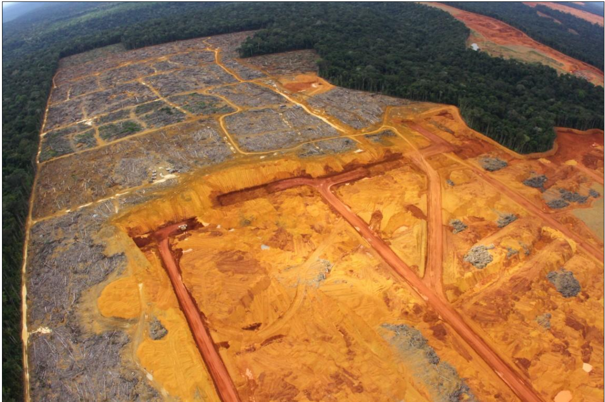
Figure 2 Relocation of Belterra Clay (yellowish material) in the strip mining of bauxite in Porto Trombetas, lower Amazon region in Brazil. Photo from Carlos Penteado. Source: Documentária Fotografia ( http://carlospenteadofotographia.blogspot.com/ ).
