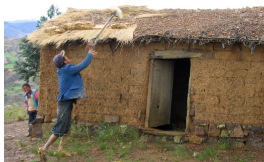
Figure 3.2 Reparation of roof cover by using woody branches, straw and loam. Photograph by R. Brandt
