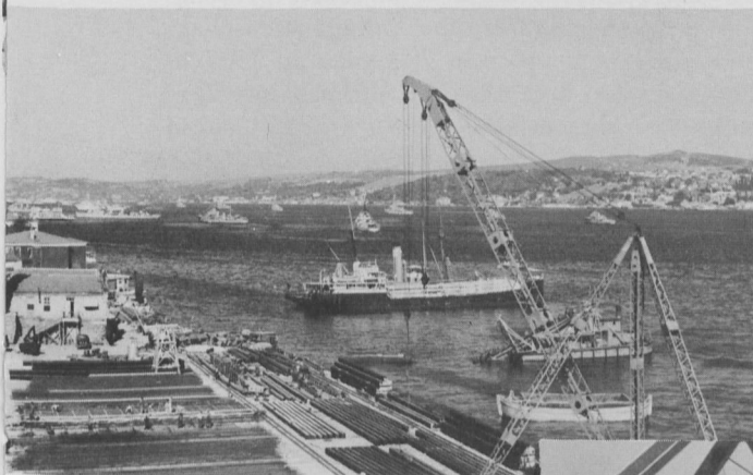
Port facilities are being expanded all along the Turkish coastline. Here is the construction of the new docks at Istanbul.
